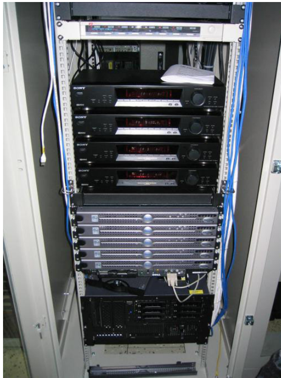
Figure 6.5: Set of tuners and servers in rack
